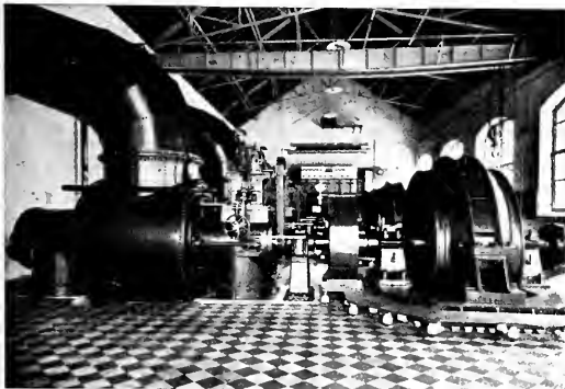
FIG. 7.—INTERIOR OF POWER HOUSE, SHOWING DRAFT TUBES.
